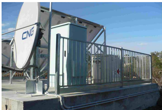
Remote power-supply back-up, using hydrogen (Australia)
