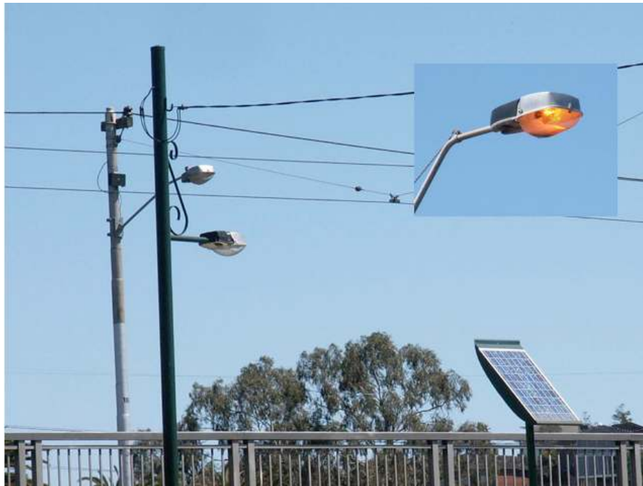
Figure 30. Example of well-meaning (or PR driven?) futile greenness – the solar panel supplies power to lights right next to the power poles. Nearby, a mains powered light burns in the broad daylight
