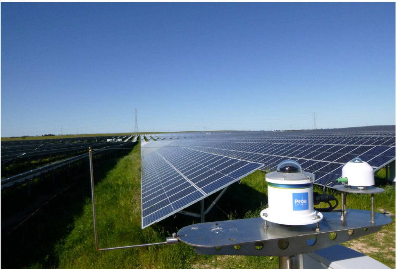
The Proa Forecasting System (PFS) installation at the 95 MW Taillem Bend Solar Project in South Australia
