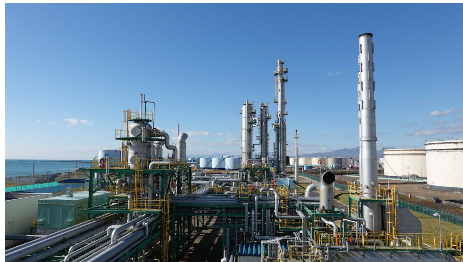
Tomakomai CCS Project, Hokkaido Island, Japan Image: IEA
