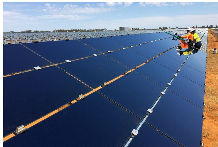
Large-scale PV: Nyngan Solar Farm
